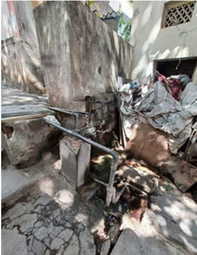
Water and Sanitation Pipelines are corroded-over a decade old and poorly managed
