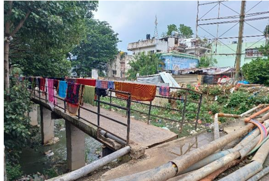
Sewerage lines regularly mix with water supply lines causing contamination and disease
